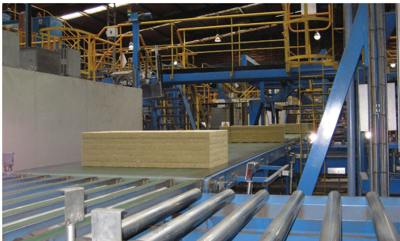
Figure 1. Atlas Copco's measurement box survey techniques were used to establish a true indication of air usage at Knauf Insulation's rock mineral wool production facility at Queensferry in North Wales.
