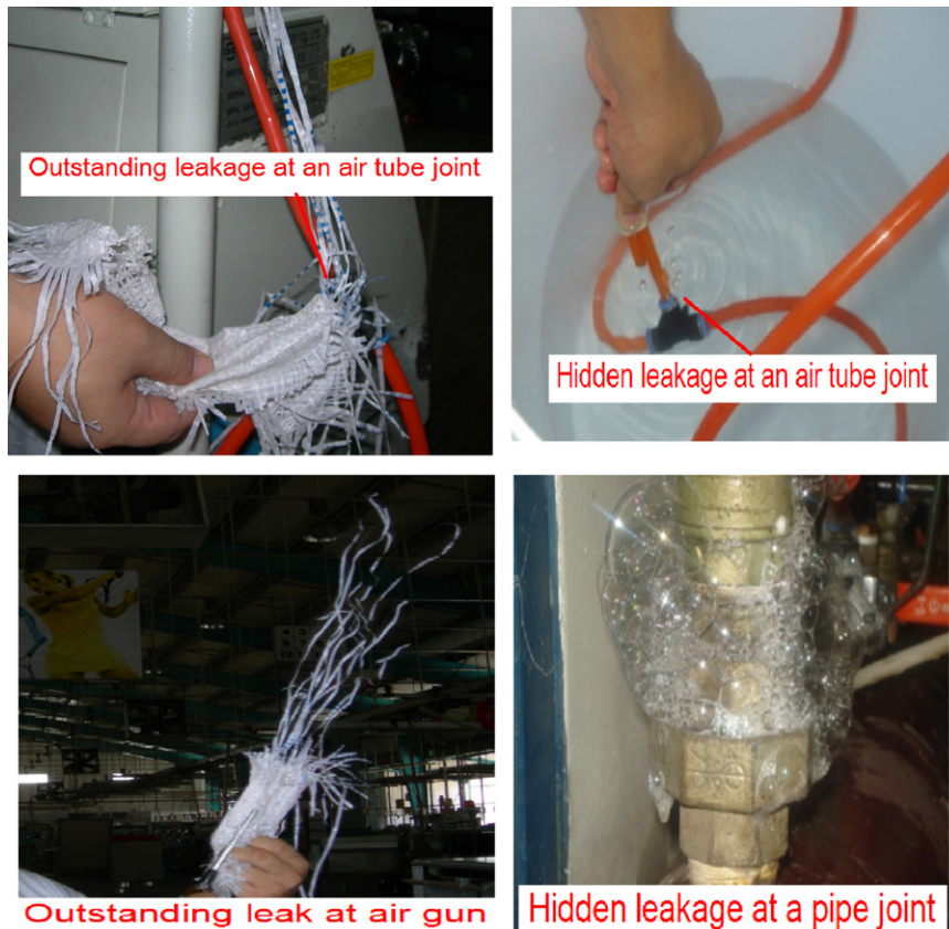
Fig. 3. Outstanding and hidden air leakages discovered in John316.
